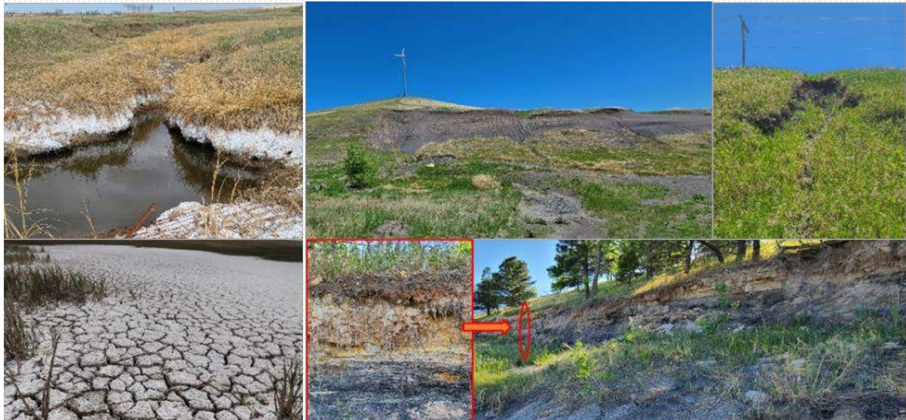
Fig. Climate Change Effects in Black Hills region – (a) desiccation cracks & salt precipitation; (b) soil erosion; (c) slope failures; (d) progressive landslide along US16
